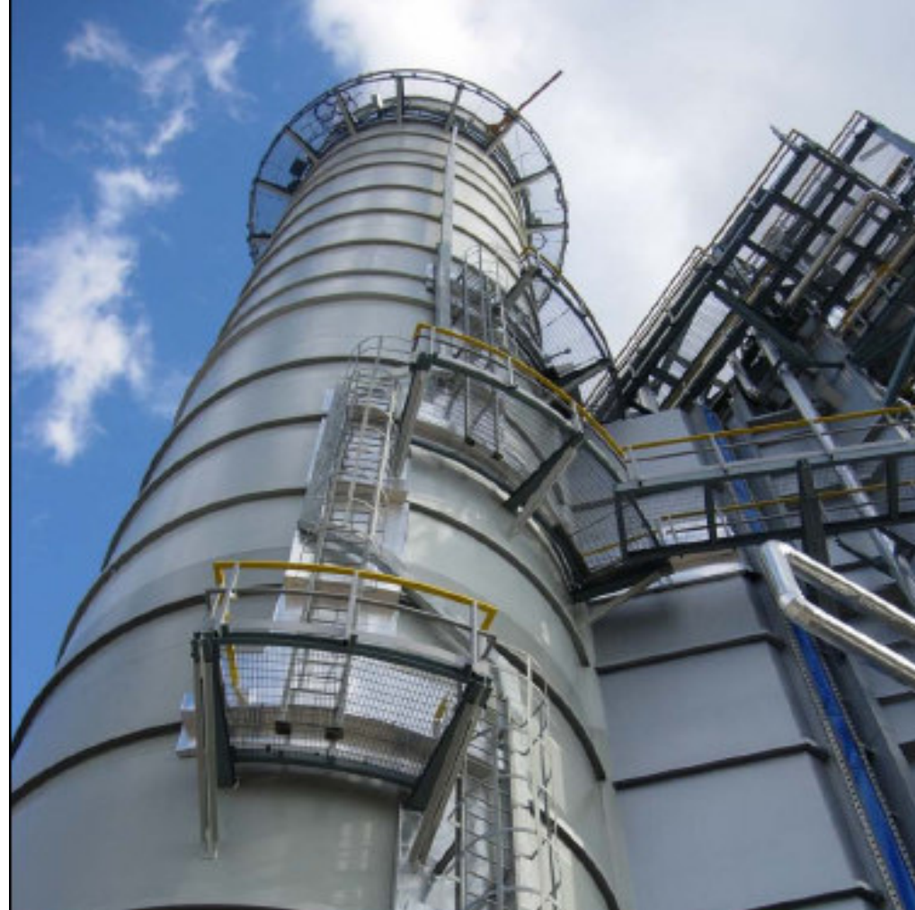
800 MW CCGT Plant in Sparanise (Campania region, Italy)
