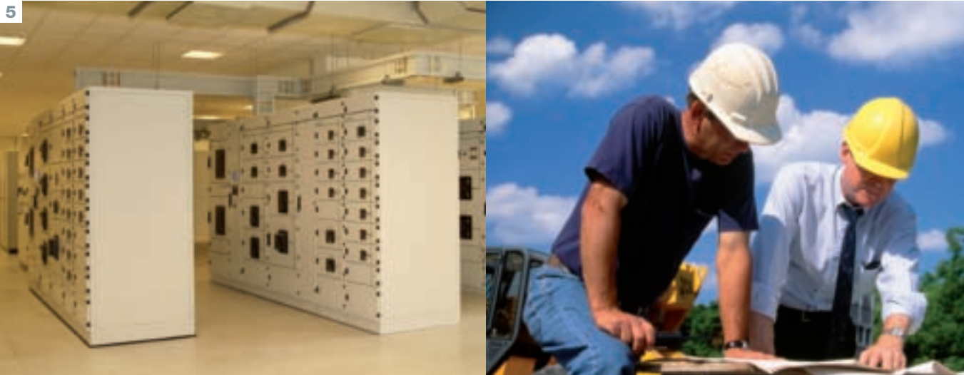
5 - Sala quadri / Electric panels room
